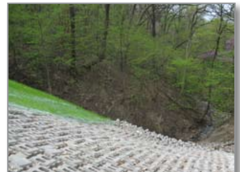
Turfgrass restoration over articulated concrete mats and interlocking concrete jacks stabilized the slopes.
